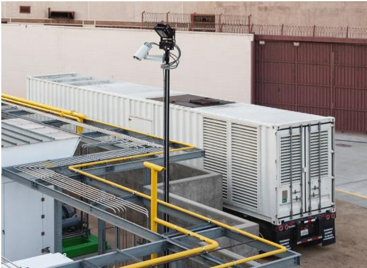
Figure 19: Backup mobile diesel generator at LA Metro Division 13, Los Angeles, CA.
