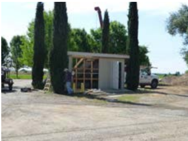
Photograph 5. View southwest of pump house.
