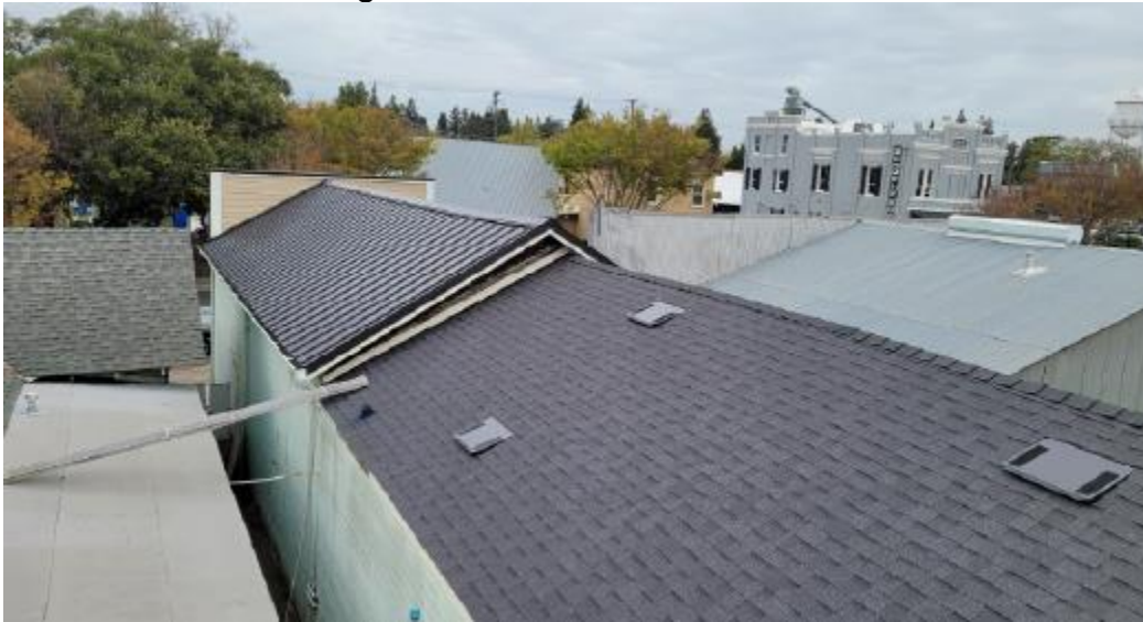
Figure 3. Reroof Current Condition
