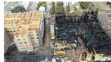
Sacramento fire officials share update on blaze that gutted Broadway affordable housing project
