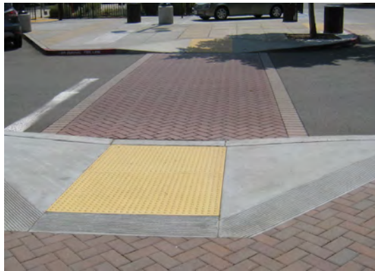
Ramp and warning strip
