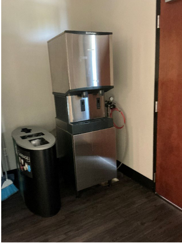
Break Room 24x73 Water and Ice dispenser with drain access
