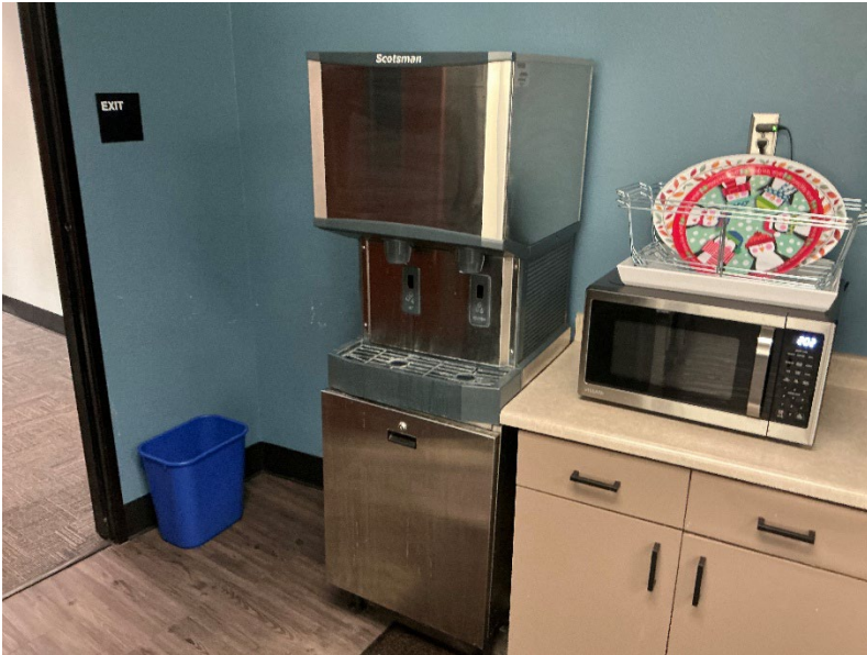
Break Room 24x68 Water and Ice dispenser with drain access
