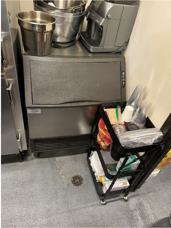
Café Elk Grove Back of House 30x26 Bin Ice Machine with drain access
