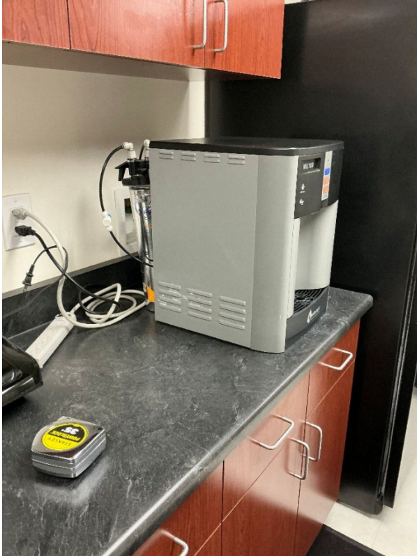
Warehouse – Portable 14x19 Countertop hot/cold water dispenser (no drain access)
