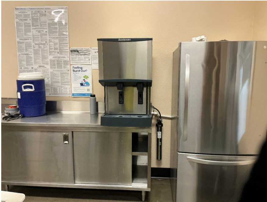
First Floor Breakroom 24x35 Countertop Ice and Water dispenser with drain to sink
