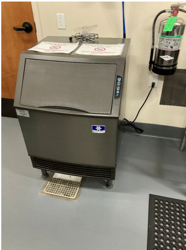
Community Center Commercial Kitchen 30x26 Bin Ice Machine with drain access
