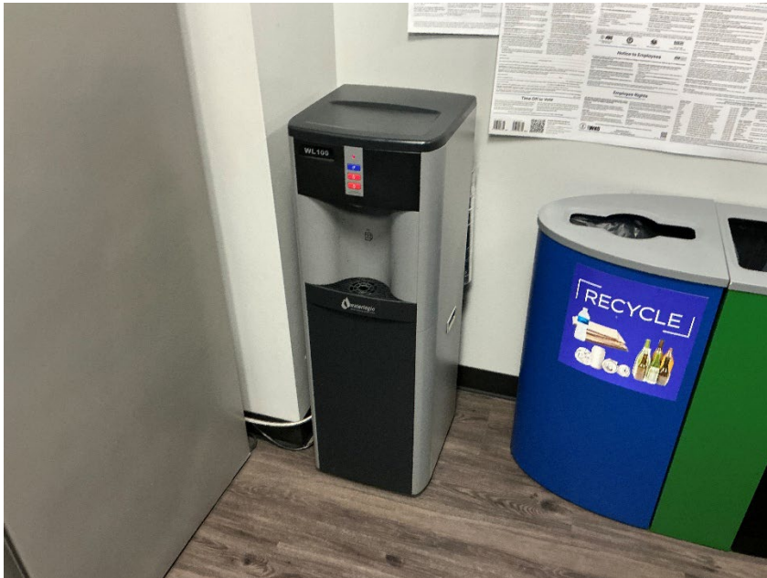
Break Room 14x41 Standalone hot/cold water dispenser (no drain access)
