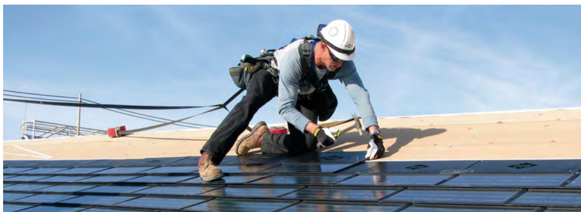
Integrated solar roof panels
