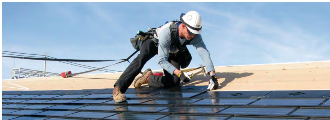
Integrated solar roof panels
